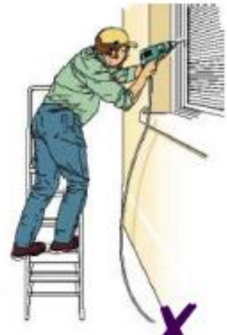
INCORRECT ✗ Steps are side-on to work activity.
